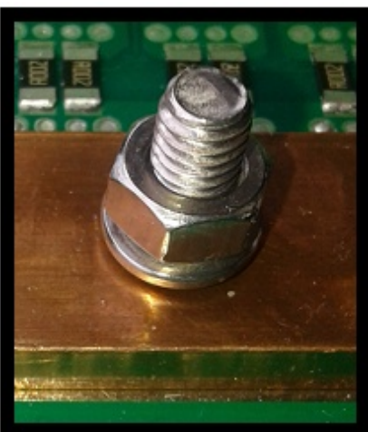
COPPER BAR BOLTS
